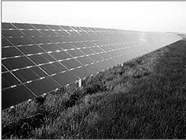
Figure 4.2 Ground-mounted solar array in the fields.
