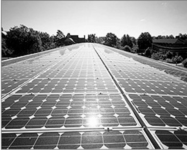
Figure 4.1 A big silicon solar array on the roof of a business.
